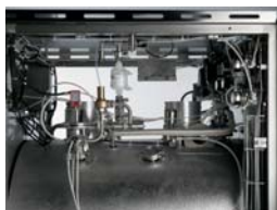
Modulating valve on steam inlet
