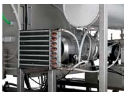
Condensate drain cooler and vacuum pump
